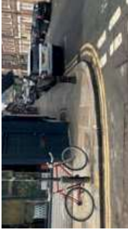
Lack of dropped kerb on Columbia Road
